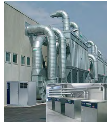
• Industrial: Pneumatic transport of wood chippings ROBOX evolution blower unit
