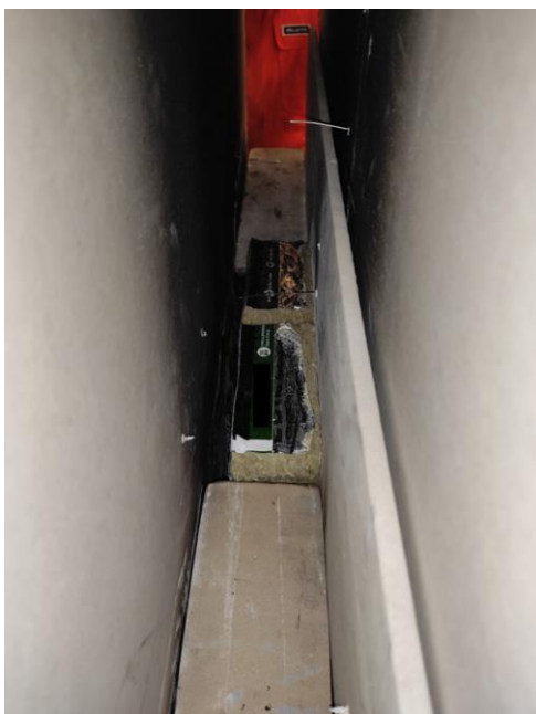
Figure 54 -Cavity barrier blocks installed within the experimental setup with a gap in between.
