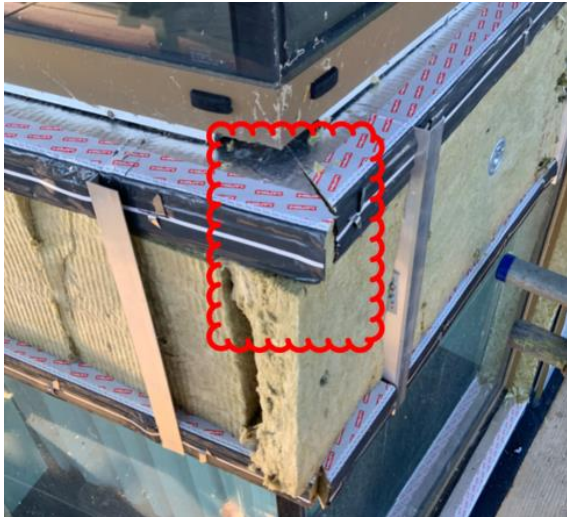
Figure 13 - Absence of intumescent strips at the corners highlighted in red cloud.
