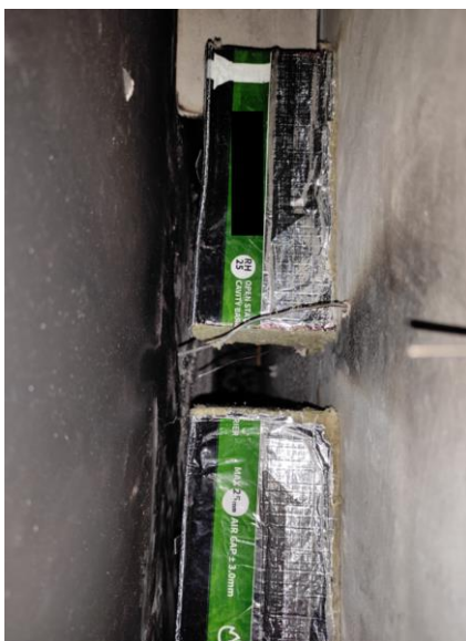
Figure 61 - Cavity barrier blocks installed within the experimental setup with a 45 mm gap in between.
