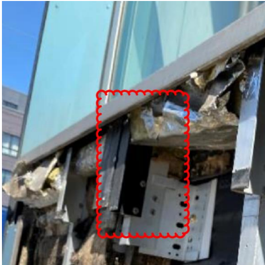
Figure 10 - Loosely packed cavity barriers with blockages in front of the intumescent strip highlighted in red cloud
