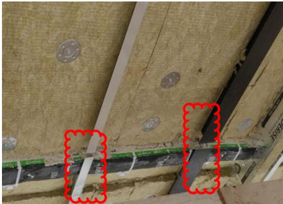
Figure 11 - Blockages in front of the cavity barrier highlighted in red colour
