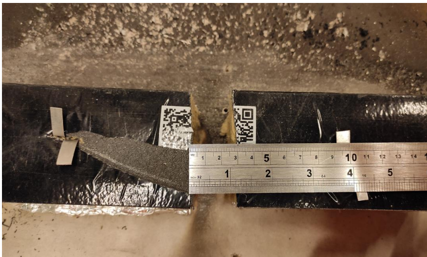
Figure 53 - Cavity barrier blocks installed over the gypsum board keeping a gap of 30 mm.
