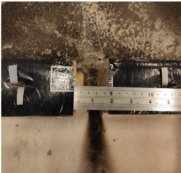
Figure 60 - Cavity barrier blocks installed over the gypsum board keeping a gap of 45 mm.
