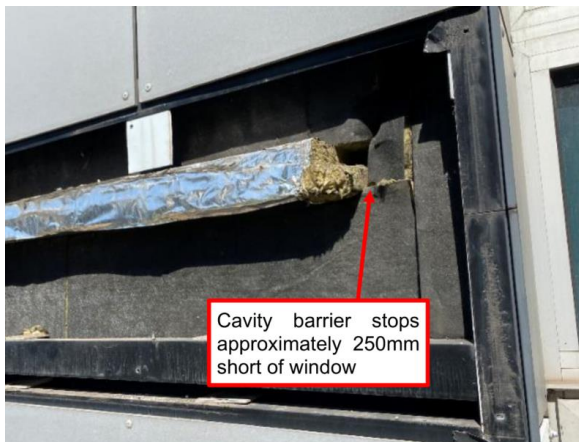
Figure 9 - Gaps or discontinuity for the horizontal open state cavity barrier
