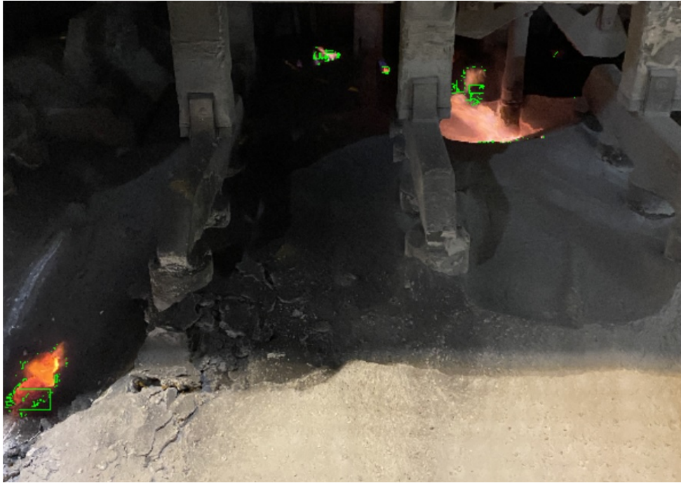
(a) Tapping hole and point flames detect as hot spots.
