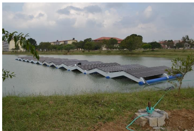
Image-1 Floating solar PV demonstration plant
