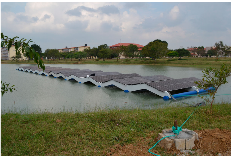
Figure 2. Floating solar photovoltaic (PV) demonstration plant. Source: University of Jaffna, Sri Lanka.
