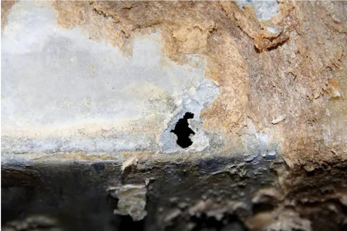
Figure 28 - Example of aluminium corrosion. (Velling, 2020)
