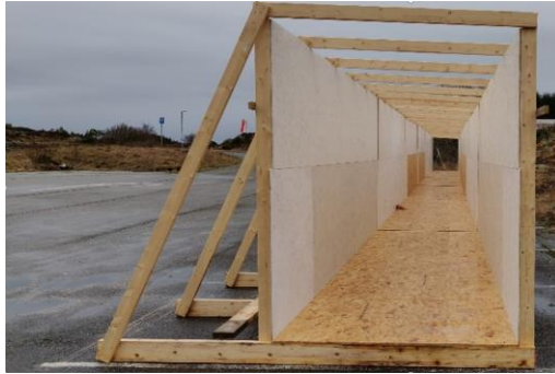
b. The Haugesund corridor fabricated from wood under construction and at 0° of heel.
