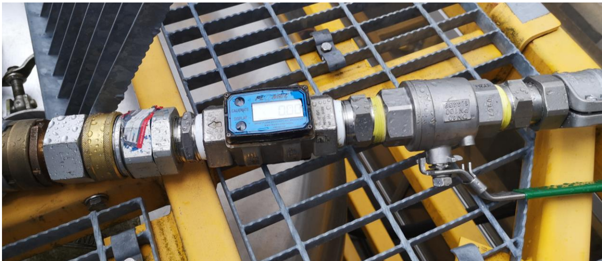
Figure 3.21 – Master flow meter
