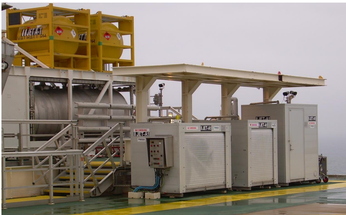
Figure 2.1 – Imenco's offshore refuelling system
