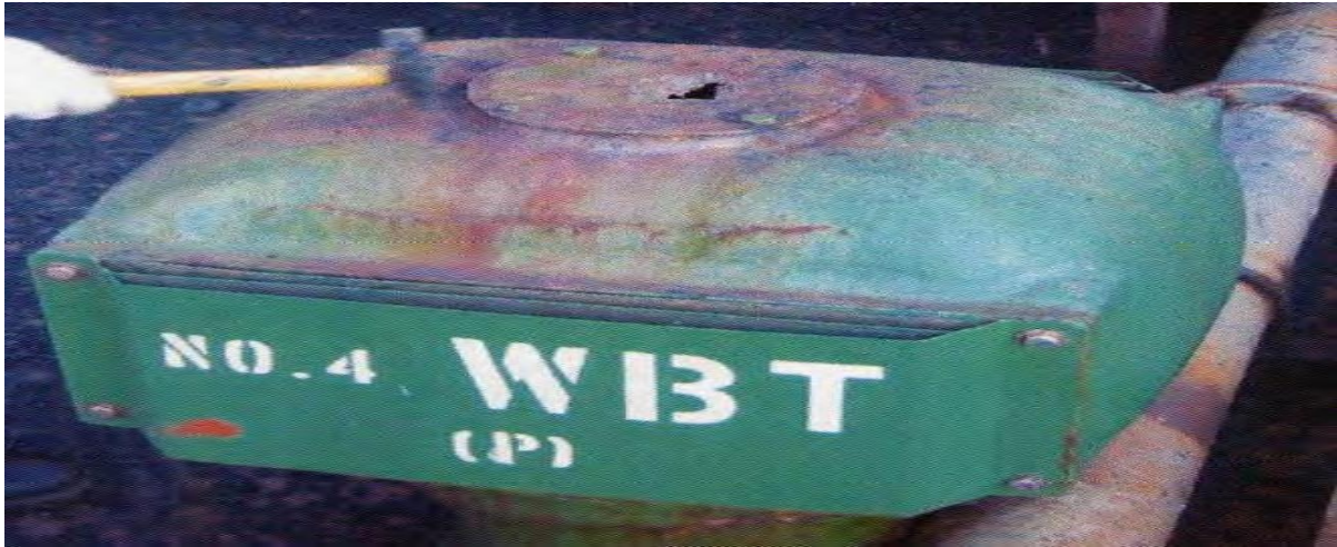
Figure 2.12: Wastage and holes of air pipe head
