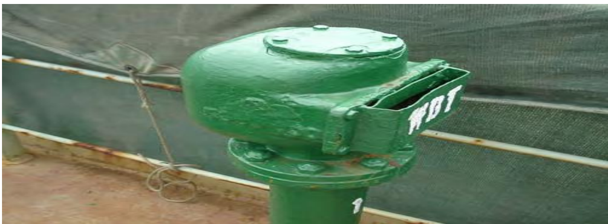
Figure 2.14: Temporary repaired by patty
