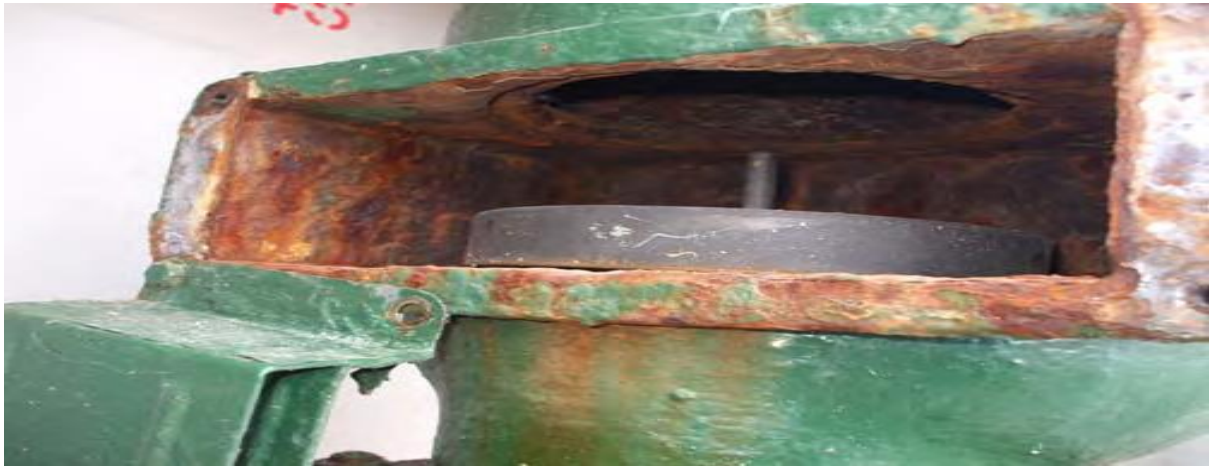
Figure 2.13: Wastage of the inside of air pipe head
