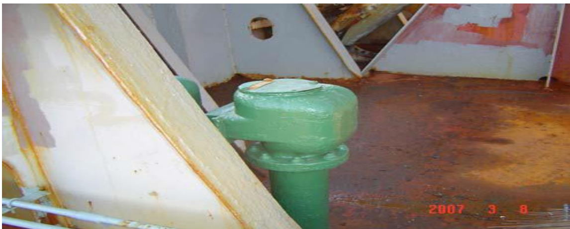
Figure 2.17: Missing bolt of air pipe head
