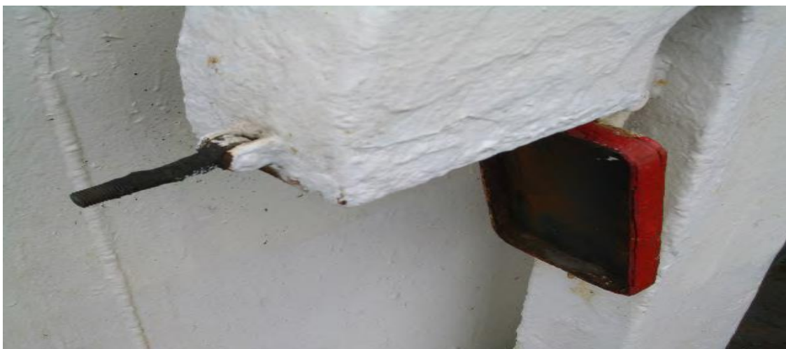
Figure 2.16: Missing butterfly nut of gooseneck ventilator
