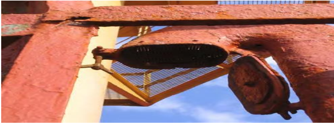
Figure 2.15: Wasted gooseneck ventilator
