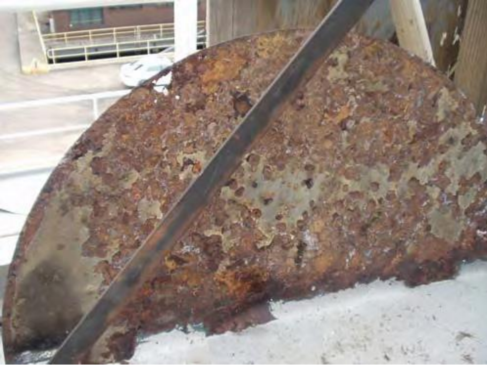
Figure 2.8: Wastage/holes in a fire damper
