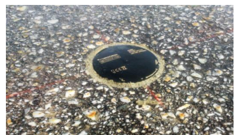
Figure 14: Installed Sensit Flush Mount
