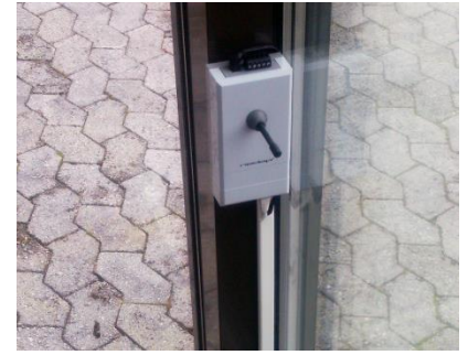
Figure 16: Installed Data Collector
