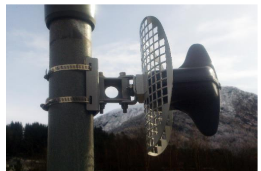
Figure 15: Mounted Relay Node, with dish
