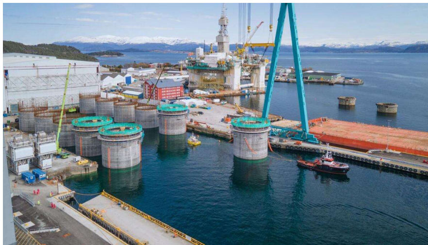
Figure A.4 The lower part of the foundations for Hywind Tampen is cast in the dock at Stord before the foundations are towed to Ålfjorden for completion (Figure from Equinor).
