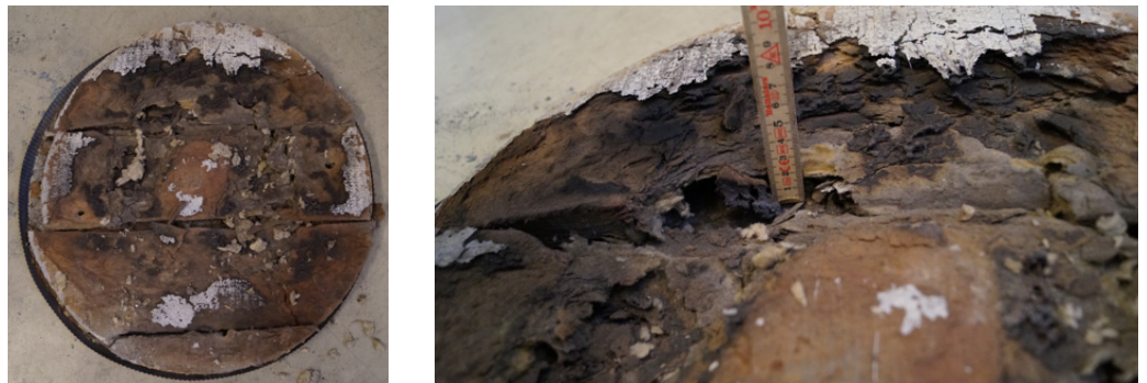
Figure 2. Thermal insulation after jet fire exposure as suggested in [19,20].
