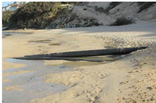
Figure 13 Cable suspension and exposure due to wave action on a sandy beach in Great Britain (Source: www.aphotomarine.com )
