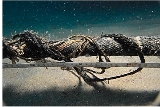
Figure 14 Abrasion failure to subsea power cable (Reda, Thiedeman, Elgazzar, Shahin, Sultan & Mckee, 2021)
