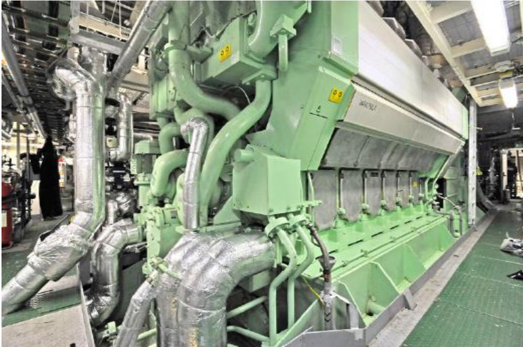
Figure 43 Engine Room in an Offshore Supply Vessel (Kopits & Losz, 2013).
