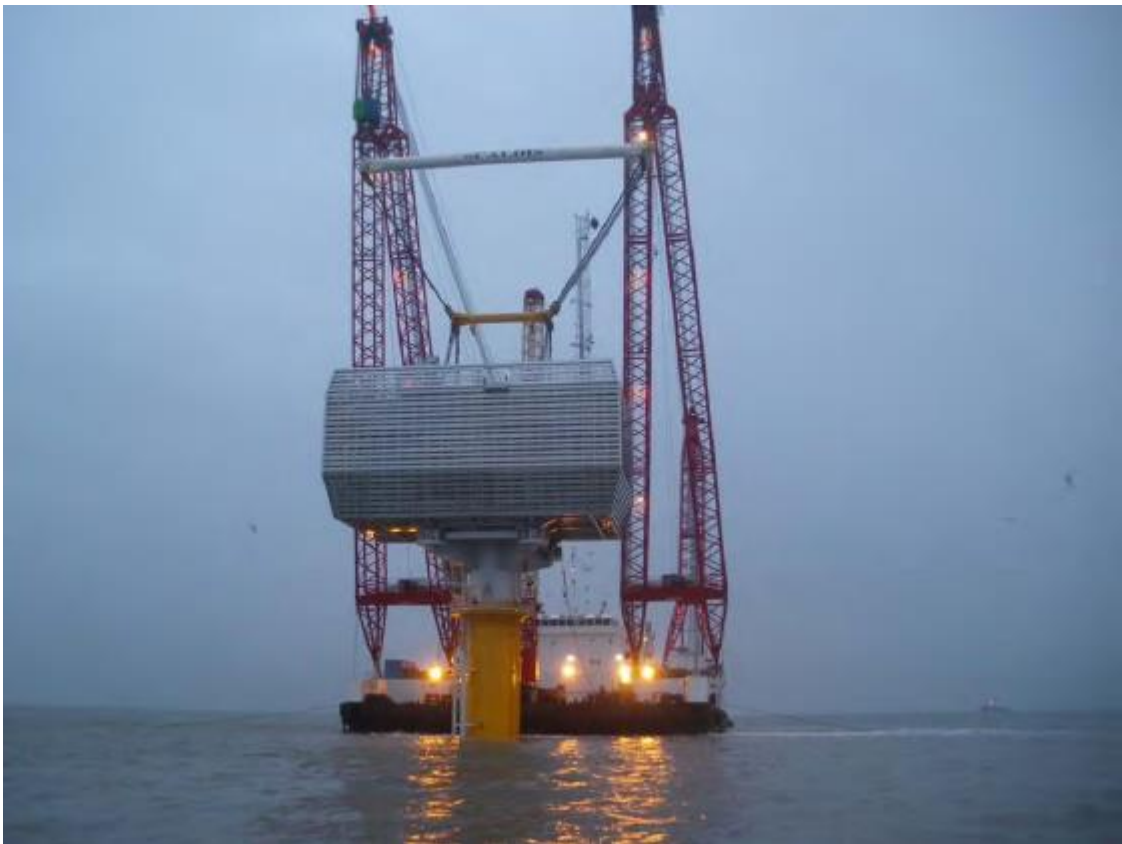
Figure 30 Substation Being Lifted onto Monopile at Gunfleet Sands (Offshore Wind Power Marine Services, 2010)
