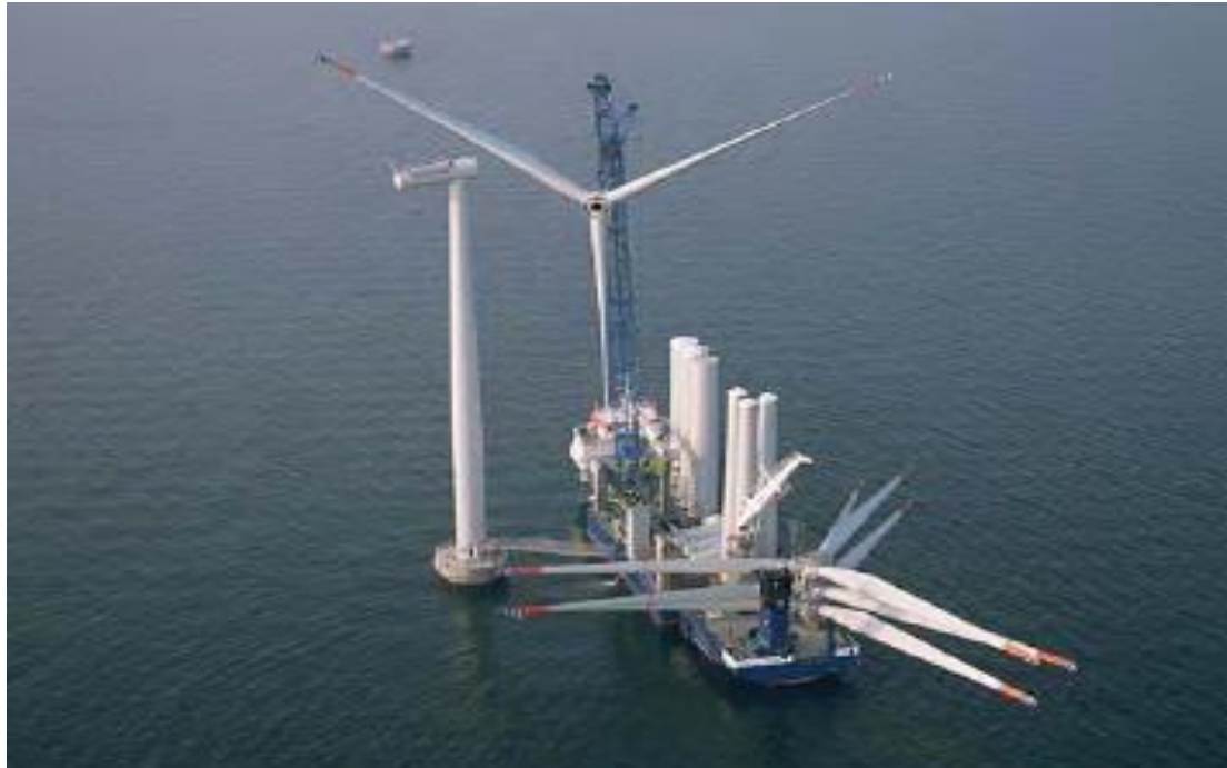
Figure 18 An Assembled Rotor Being Lifted onto a Nacelle at Nysted (DONG Energy 2010a as cited in (Kaiser & Snyder, 2010)
