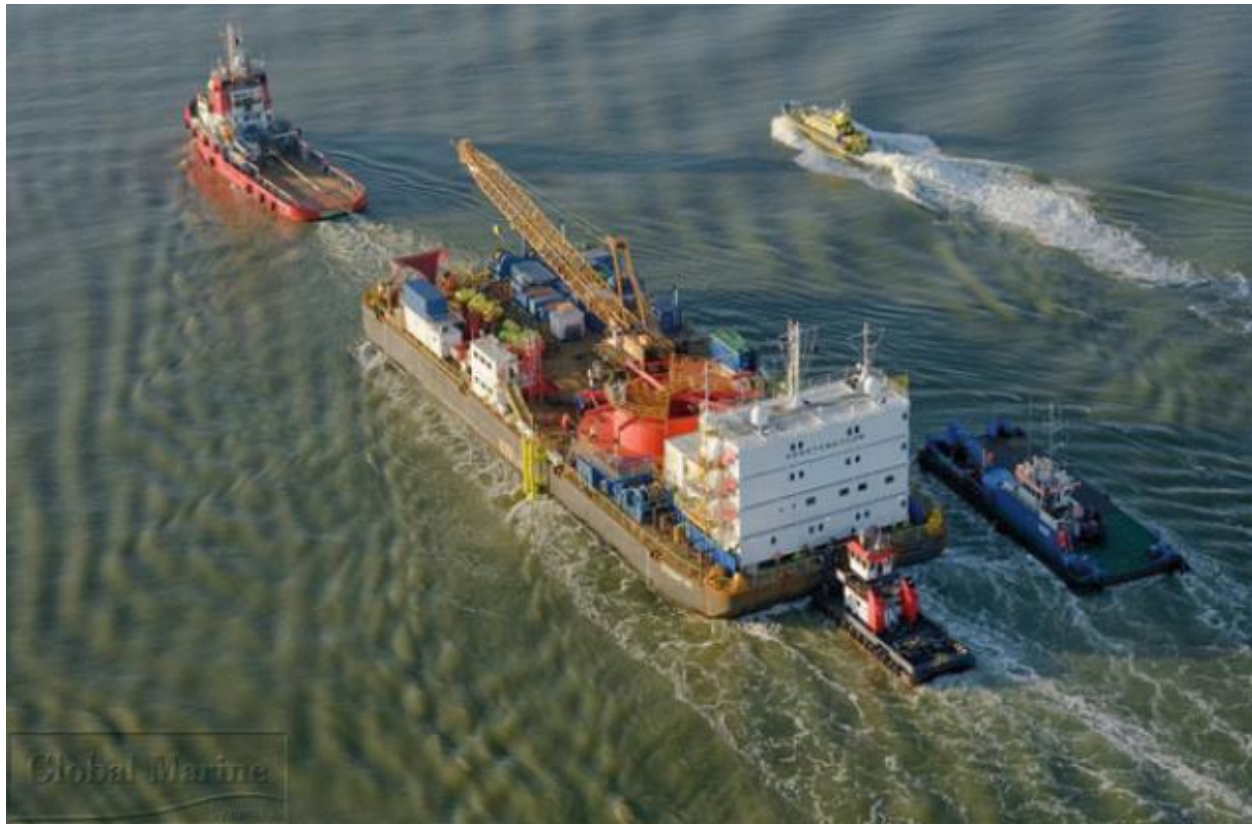
Figure 29 Cable laying barge with spread (Global Marine Systems, as cited in Kaiser & Snyder, 2012)
