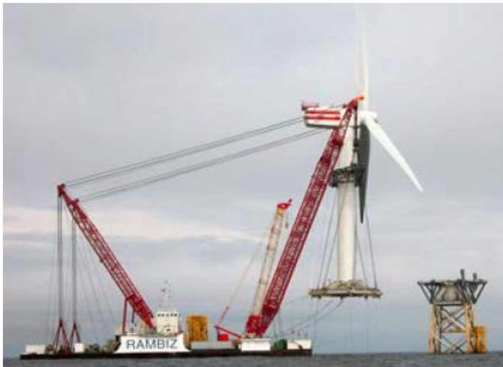
Figure 37 Rambiz Installing a Wind Turbine at the Beatrice Wind Farm (Kopits & Losz, 2013).
