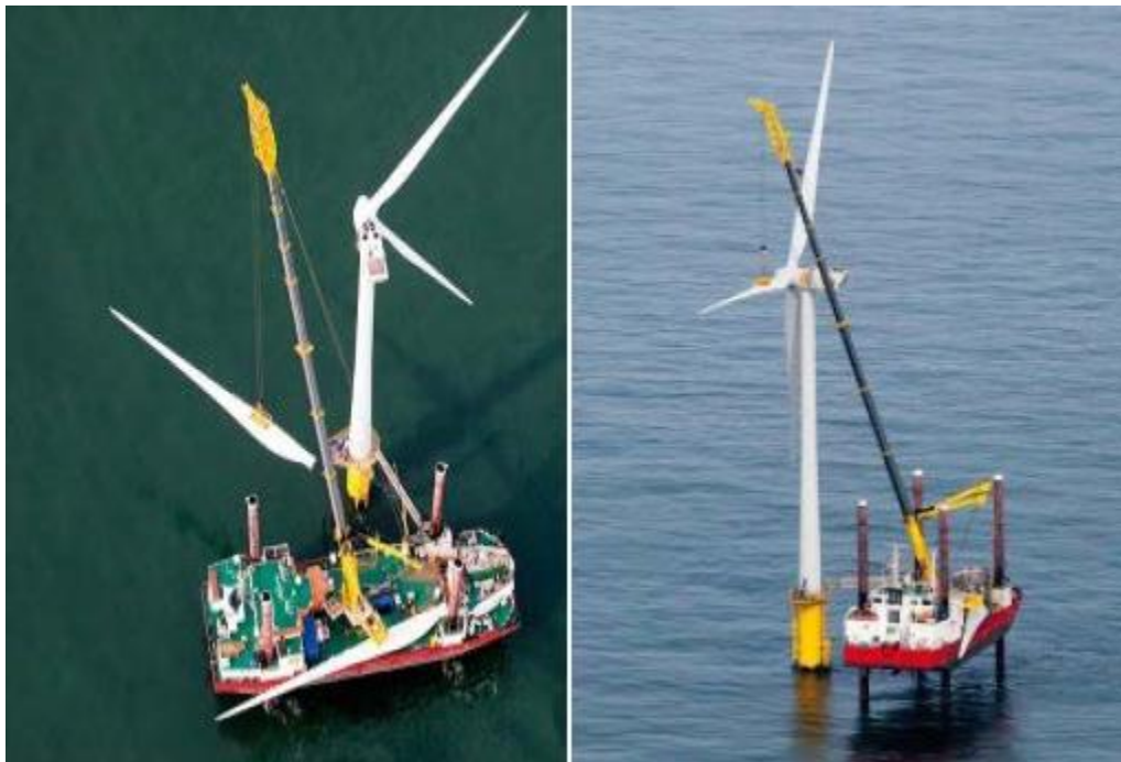
Figure 38 MV Wind Installing a Nacelle Using a Lattice Boom at a Dutch Wind Farm (Kopits and Losz, 2013).
