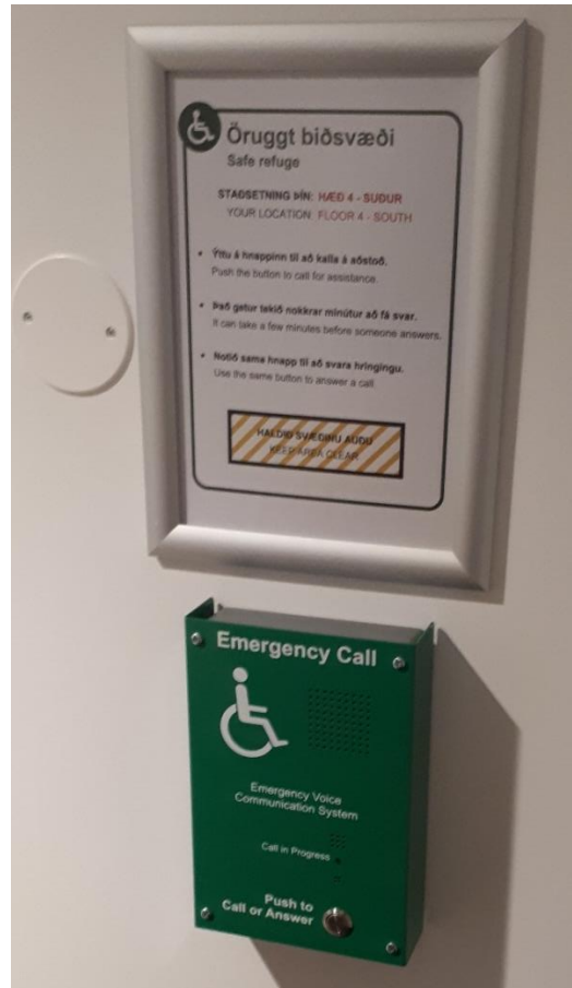
Figure 17: Communication device in refuge area (Picture taken in evacuation exercise)
