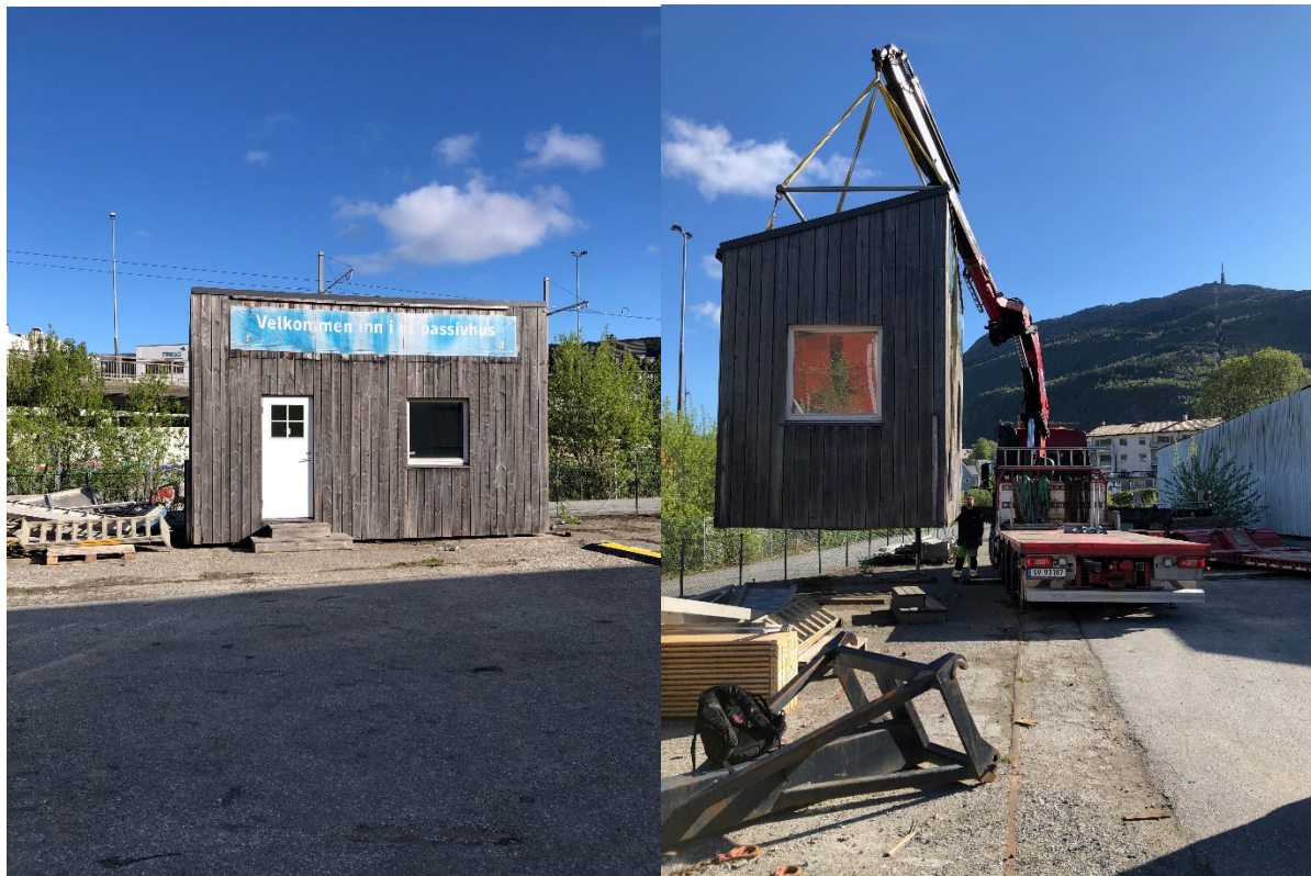
Figure 17 To the left, the passive house in its initial location
