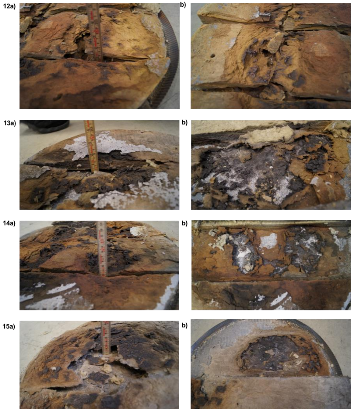
Figure I. 12 12 a and b) Insulation after test 12. 13a and b) insulation after test 13. 14a and b) Insulation after test 14. 15a and b) Insulation after test 15.
