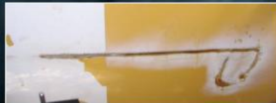
Subsea Pipeline surface damage (above) and 3D rendered laser model (below)
