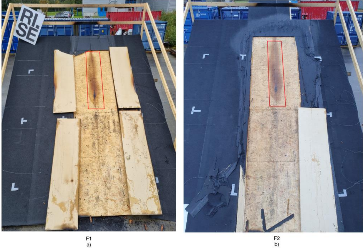
Figure 45: Marks from burn-through at the joint of the chipboards in experiment F1. The burn mark did not increase further after experiment F2
