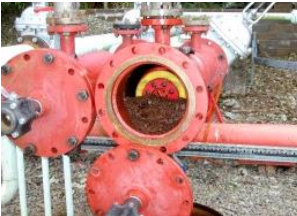
Figure 10: Debris after pigging operation [18]
