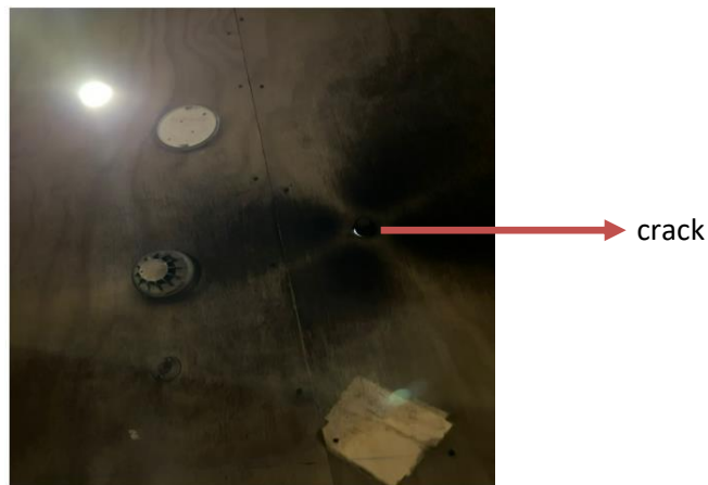
Figure 12: Crack on the ceiling
