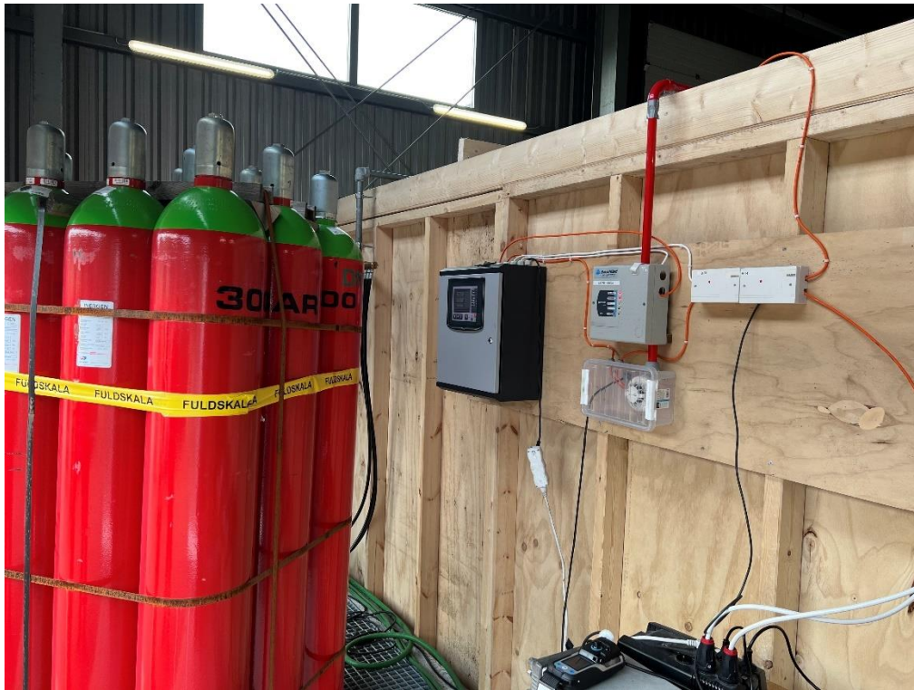
Figure A7: Inergen gas extinguishing system with Alarm control panel, Aspiration detection unit and Boxed chamber for multi-sensor detector
