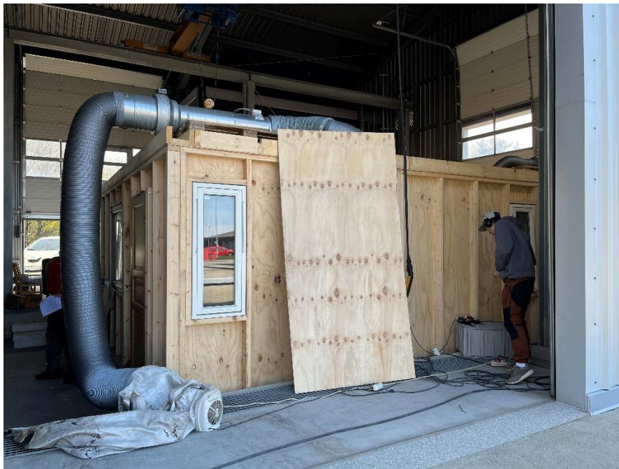
Figure A10: Ventilation System of test apartment
