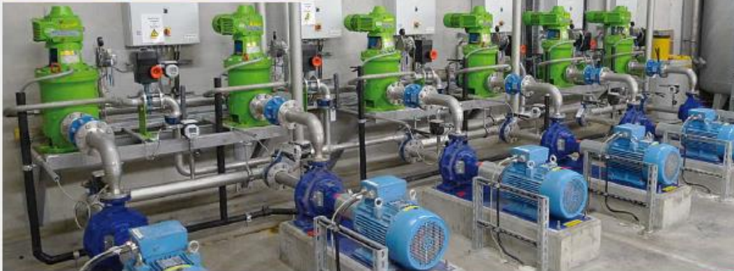
Fig. 4 sealing water filtration in power plant
