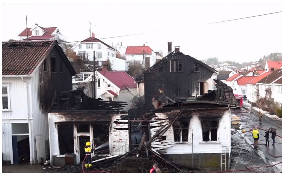
Fig. 11. Three buildings lost in fire 24 February 2014, Risør historic village, Norway. (Photo by Hans Petter Bjerva. Reproduced with permission).
