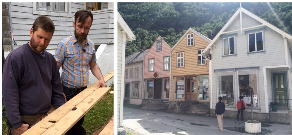
Fig. 5. Deep burn marks in the roof construction discovered when refurbishing a roof (on the pink house) in Old Lærdalsøyri, July 5th 2016. (Photo: Odd Helge Brugrand/NRK. Reproduced with permission.)
