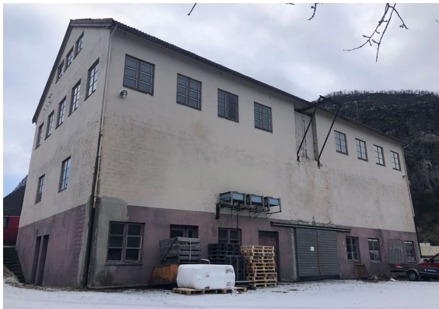
Figure 6: The existing building seen from north. Source: taken by the author January 26, 2021.
