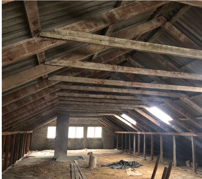
Figure 7: The existing roof seen from the attic. Source: taken by the author January 26, 2021.
