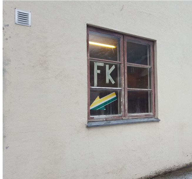
Figure 8: Existing window on the north-east wall. Source: taken by the author January 26, 2021.
