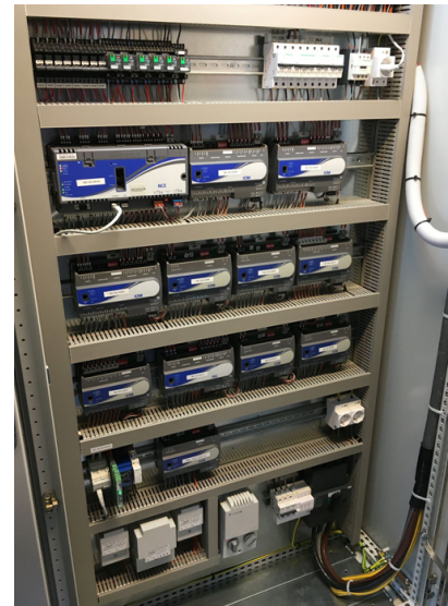
Figure 13: Cabinet housing PLC units for a propane based heat pump system. Picture taken from the field work at our reference system location.
