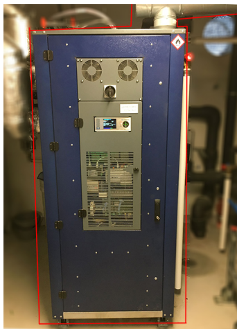
(a) EX enclosure with an exhaust line in upper right corner
