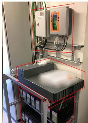
(b) Propane sensor head unit, UPS and a battery bank
