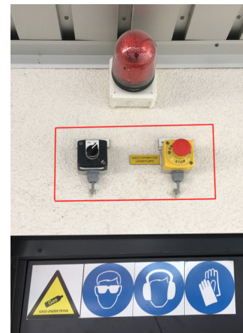
(c) Manual controls situated outside of the room
