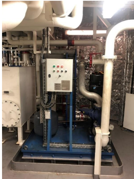
Figure 24. The Anchor Winch cooling system.
