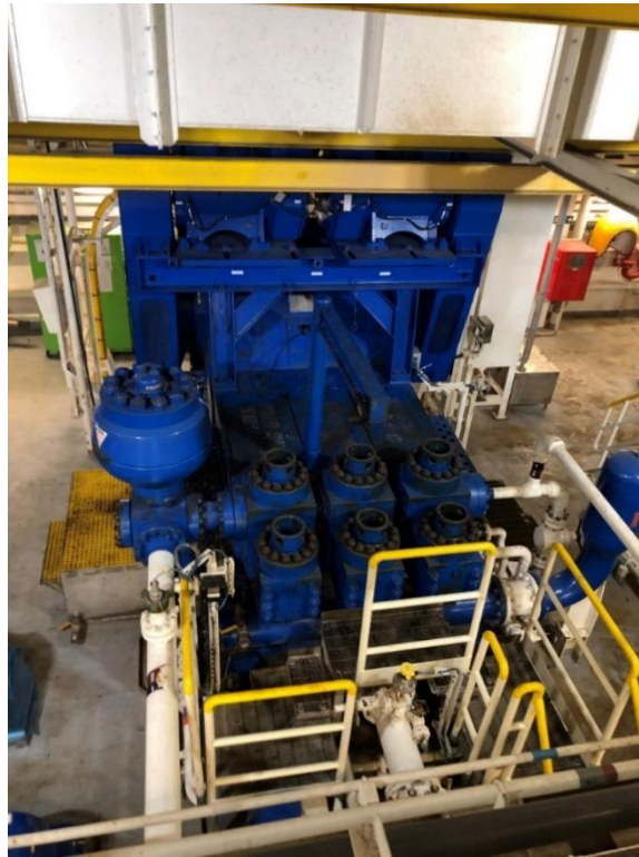
Figure 25. One of four Mud Pumps.
