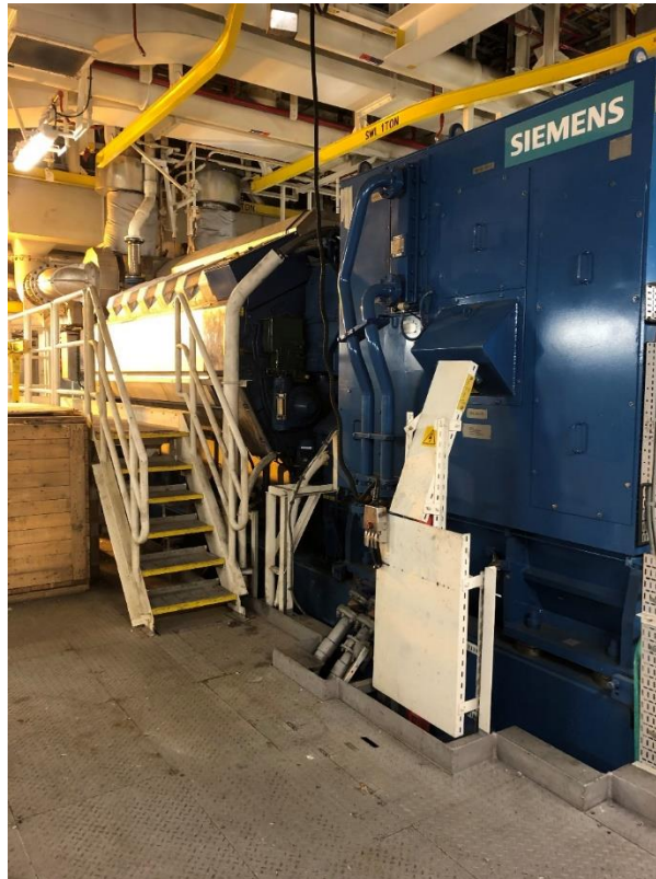
Figure 51. Engine and generator
