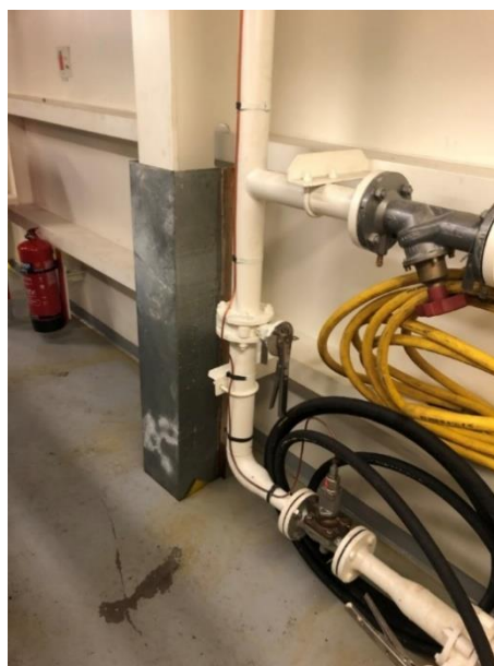
Figure 26. Automated valve and bypass for WCCU.
