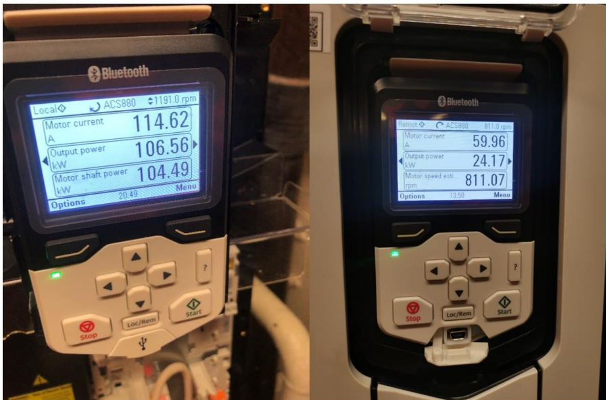
Figure 37. Power consumption before (left) and after (right) implementing pressure regulator.
