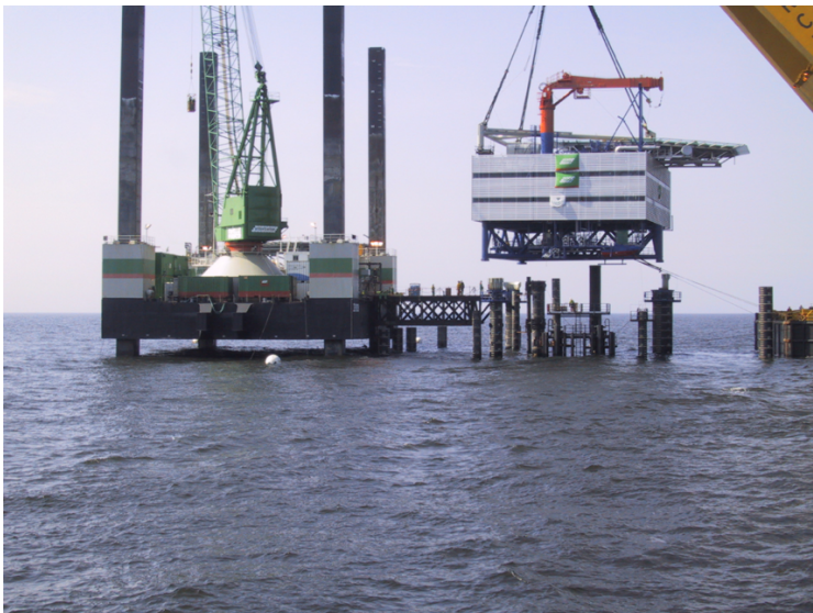
Fig. A.3: Horns Rev 1 Substation a, b, and c (Source: HSM Offshore, 2002)
