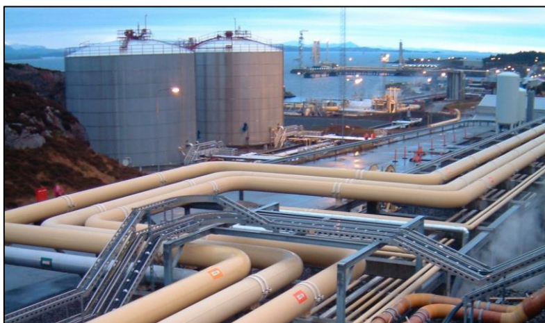
Figure 1.1 - The Sture Terminal Photo: (Equinor, 2021)
