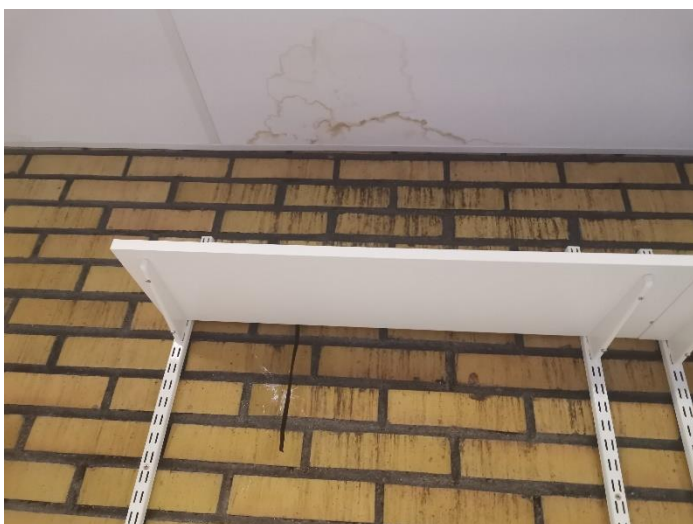
Figur 424 Fuktskade i himling i gang, plan 1
