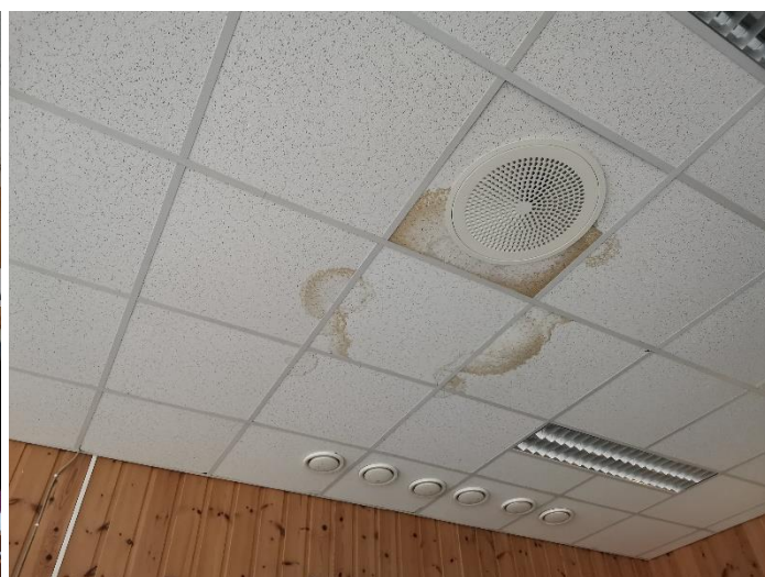
Figur 510 Fukt i himling
