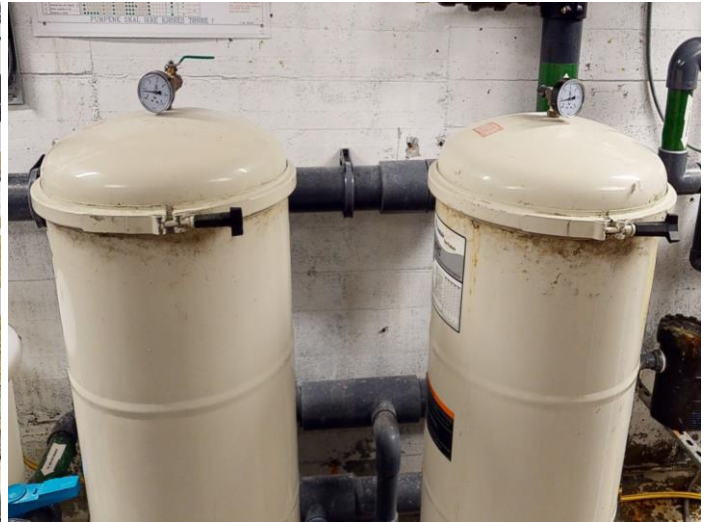
Figur 404 Reinsketank i bassengkjellar
