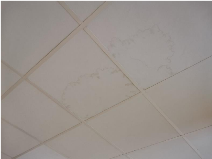
Figur 425 Fuktskade i himling i kantina, plan 1
