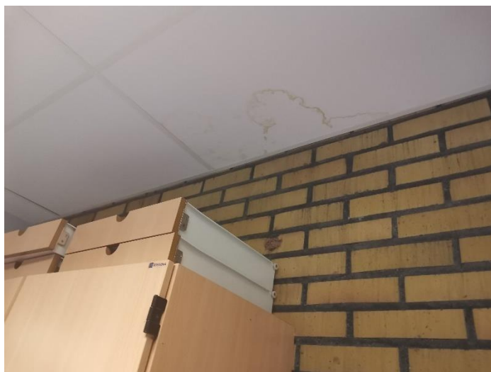
Figur 422 Fuktskade i himling i gang, plan 1
