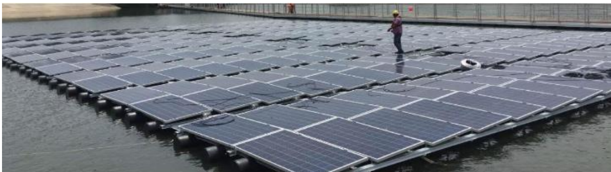
Figure 1 - Upsolar/SolarMarine Energy FPV array in Singapore
