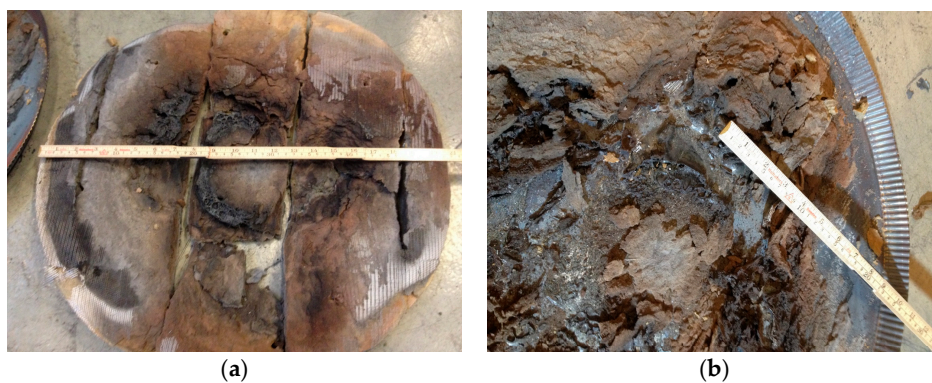
Figure 13. (a) Upper part of exposed thermal insulation after Test 2 and (b) lower part thermal insulation after Test 2.
