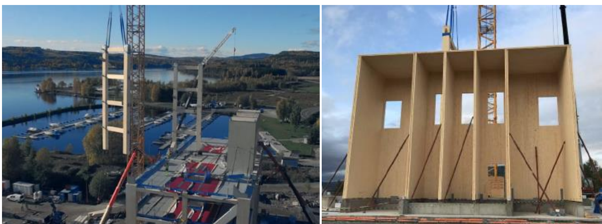
Figure 46 Construction site of the Mjøstårnet project. Installation of the pre-assembled Glulam structure and CLT shafts [61]
