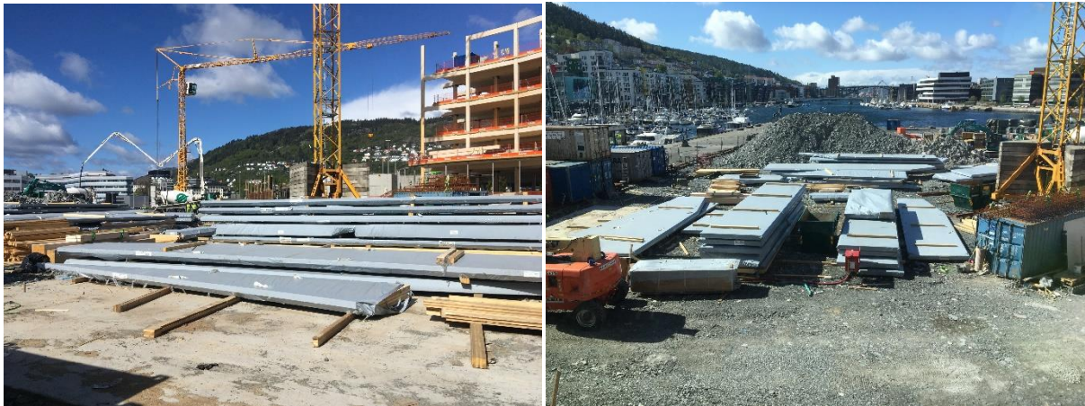
Figure 43 Construction site of the Skipet project in Bergen, material storage location and crane handling
