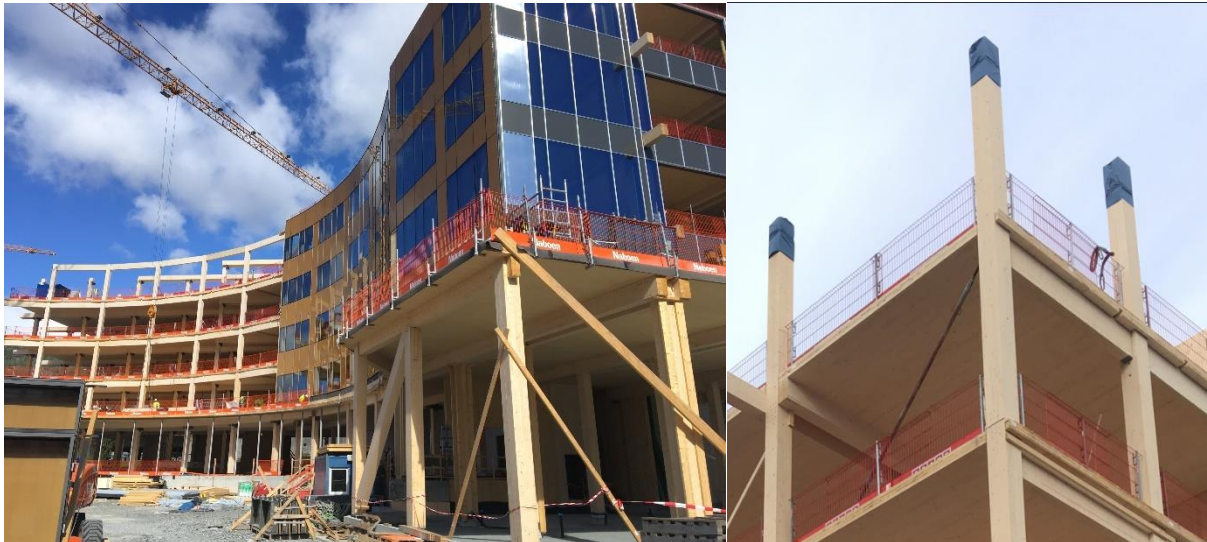
Figure 41 Construction site of the Skipet project in Bergen. Half of the building is enclosed (right). Protective tarpaulin covers give protection to the end grain of the panels and columns [by author]
