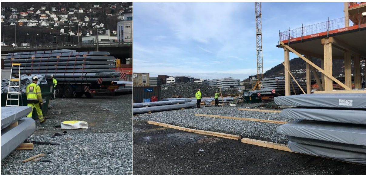
Figure 42 CLT and Glulam elements on-site delivery, routine checks and preparation for on-site storage of elements [by author]
