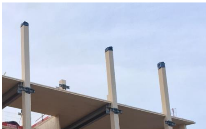
Figure 39 Waterproof tarpaulins used as end-grains protection on Glulam columns, while construction – Project: Skipet [by author]
