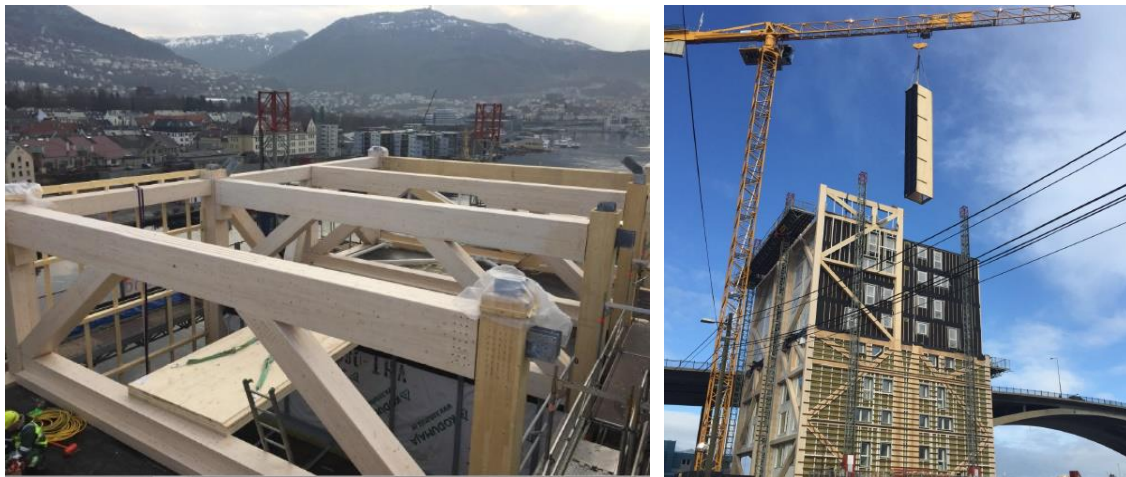
Figure 52 Protective plastic covers give protection to the end-grains of the Glulam columns (left). Installation of CLT elevator shafts (right) [63]
