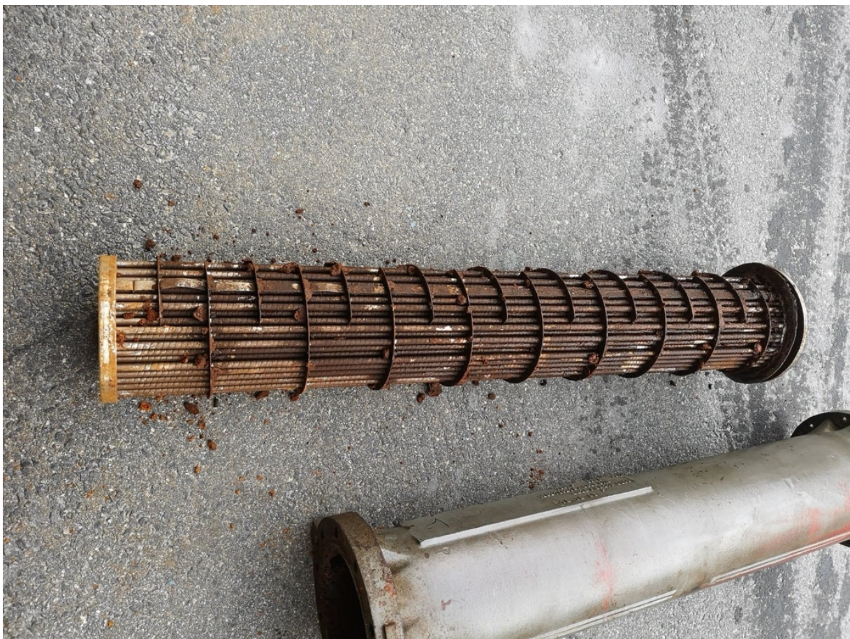
Picture 2 An example of a polluted cooling system, it is usually worse.
