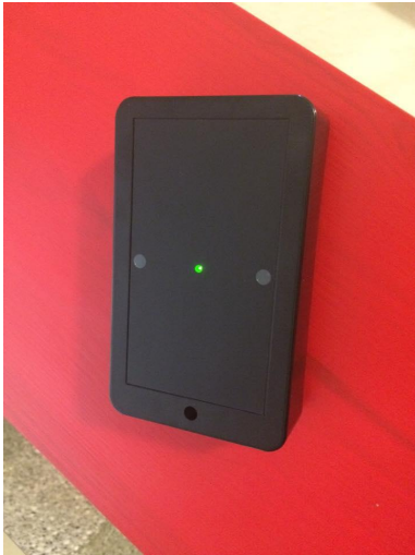
Figure 3: Receiver at intervention stairs, close-up.
