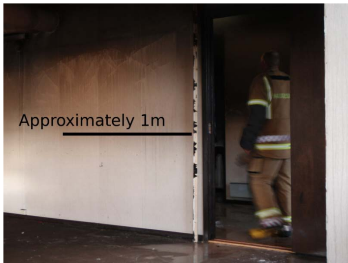
FIGURE 31: PICTURE TAKEN FROM CLASSROOM PART 3, VIEWING THE WALL SEPARATING IT AND THE HALLWAY. SMOKE-STAINS ARE CLEARLY VISIBLE DOWN TO APPROXIMATELY 1METER.
