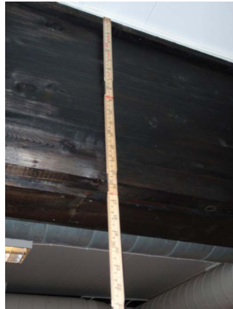
FIGURE 3: ONE OF THE BEAMS IN THE CEILING, THIS ONE IN THE START ROOM. THE EXTENSION BELOW THE CEILING IS 40 CM.
